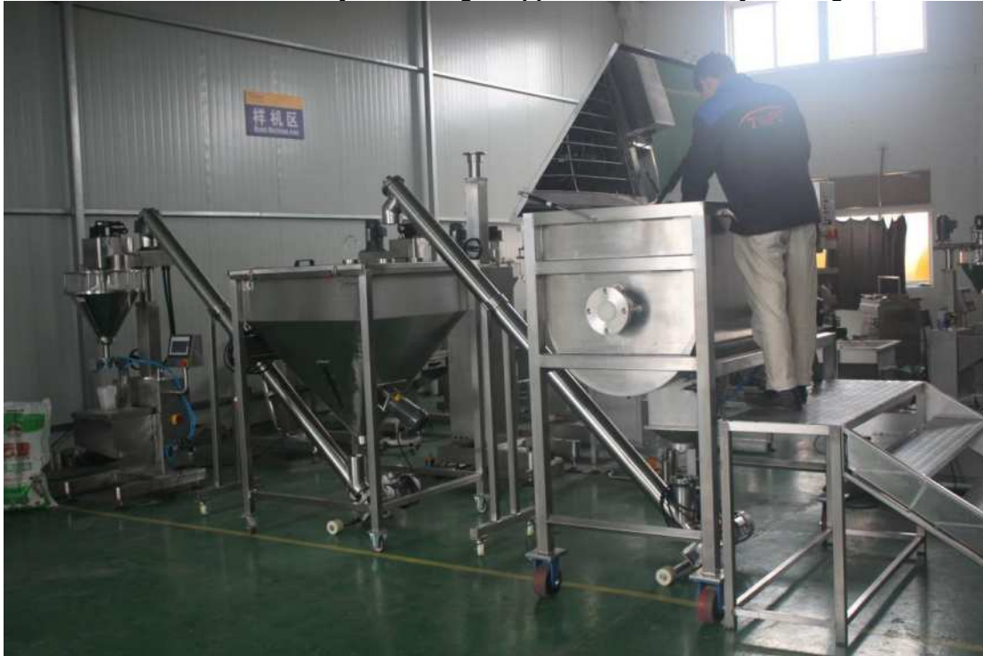
3, ribbon mixer + screw conveyor + storage hopper + screw conveyor + auger filler
